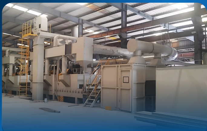
Automatic Shot Blasting, Painting & Drying Line for Steel Plates and Structural Steel
