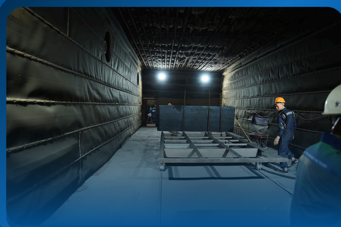
Abrasive Blasting Booth
